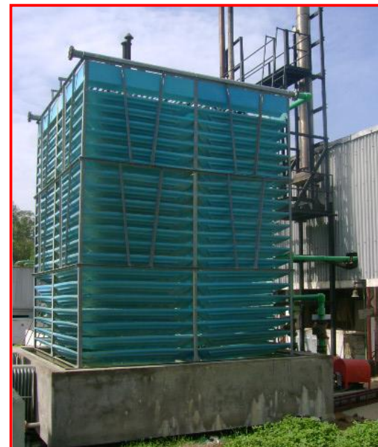
Cooling tower without fan
