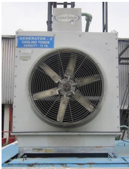
Cooling tower with fan
